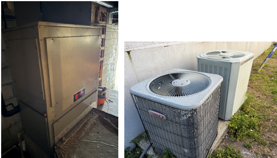
Theater 1 HVAC System
