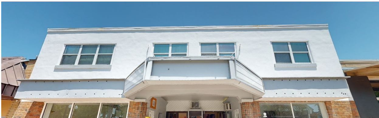
Image 27: Structurally failing marquee sign.
