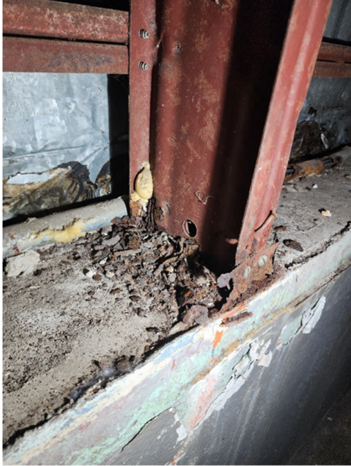
Image 6: Fully deteriorated base of Quonset frame connection.
