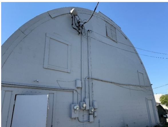
Existing electrical service
