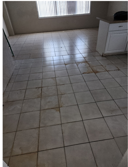
Image 14: Tile sloping in Apartment 2
