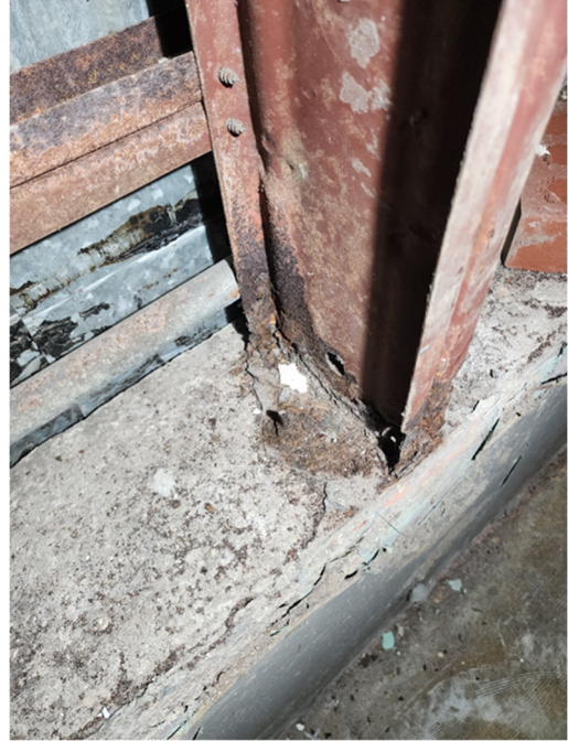
Image 7: Fully deteriorated base of Quonset frame connection.
