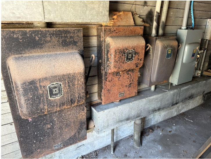
Service disconnects & wireway
