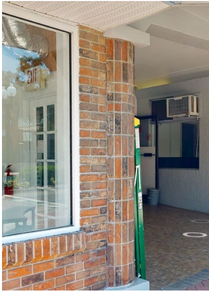
Image 5: Left column mortar joint line connection to facade.
