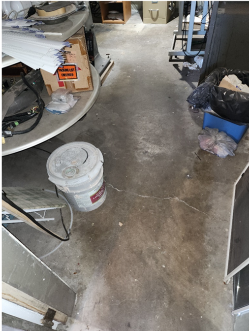
Image 13: Slab crack in Projection Room 2
