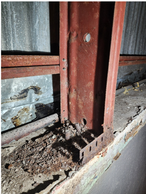
Image 3: Fully deteriorated base of Quonset frame connection.
