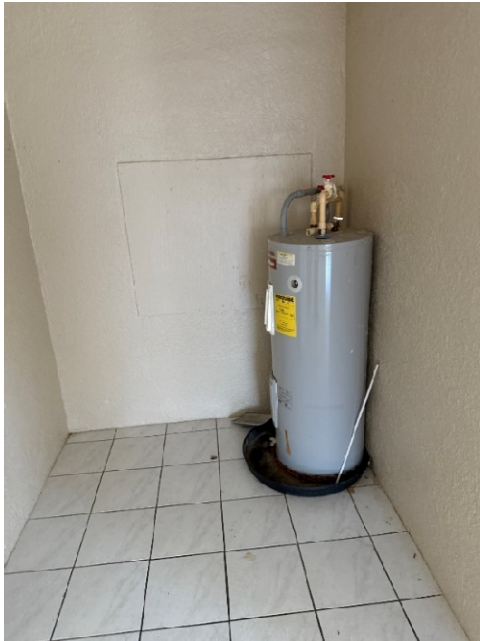
Tank water heater for apartments.
