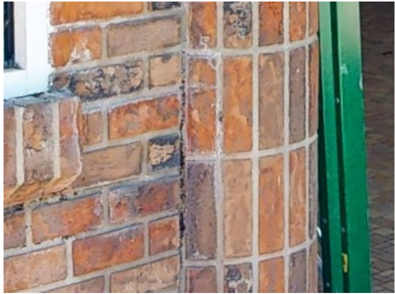
Image 6: Biological growth in mortar joint.
