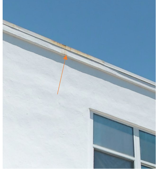
Image 22: Rusted, damaged roof flashing.
