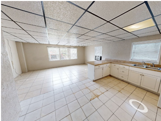
Image 42: Current condition of both apartments.
