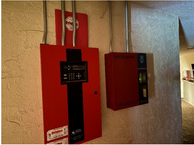
Fire Alarm Control Panel
