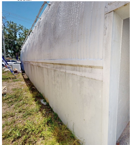
Image 18: Failing stucco and CMU Quonset Hut.
