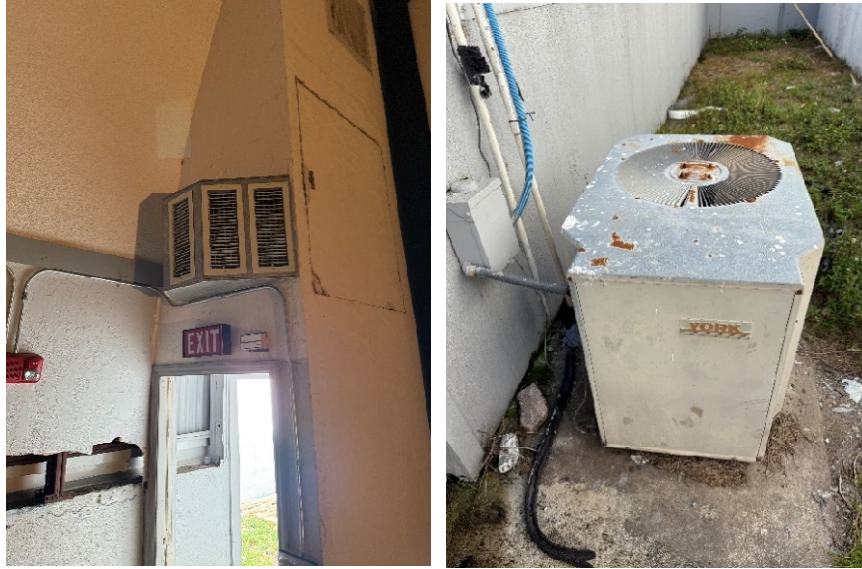
Theater 2 HVAC System
