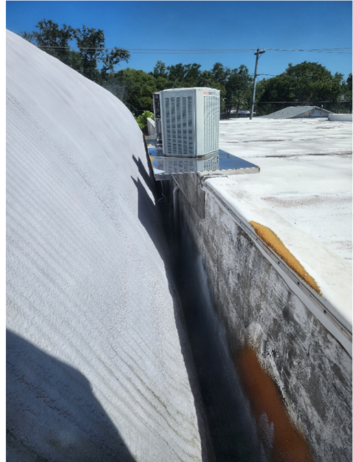
Image 2: East Wall of Quonset Hut. Roof Drainage problem area.
