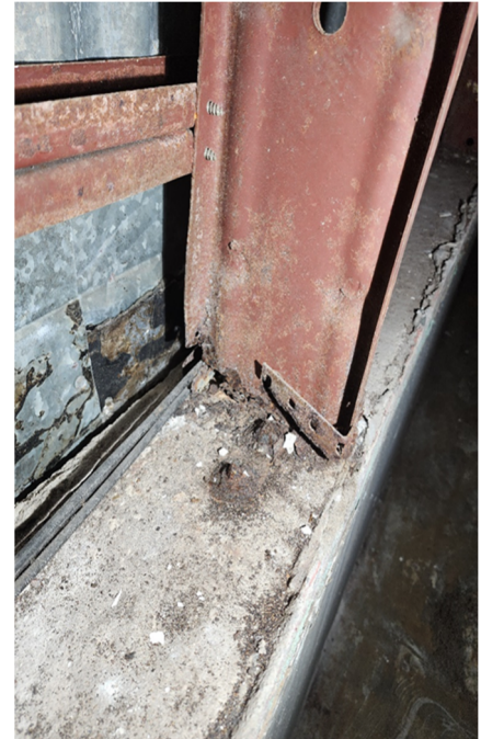
Image 5: Fully deteriorated base of Quonset frame connection.
