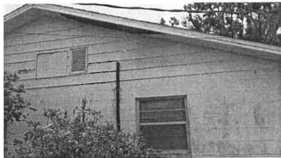
Close-up view of damaged soffits on side elevation
